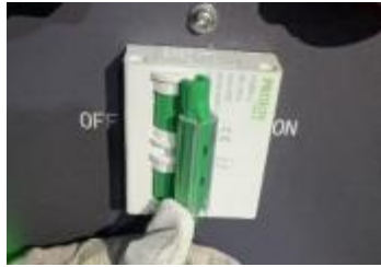
Turn on the battery main switch
